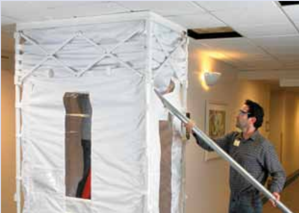
▼IMAGE 7: ECU2 containment. Disposable envelopes can be used on the frame and modified to seal off the work area within the ECU2 envelope
