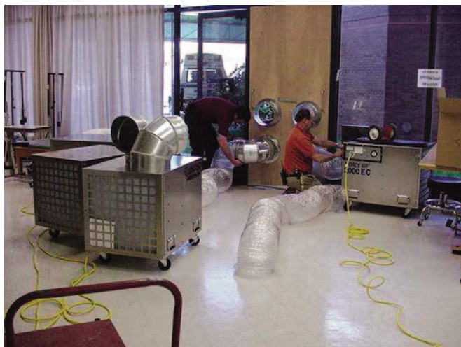
Figure 2. Photograph of HEPA filtered forced air machine installation with door insert already in place.
